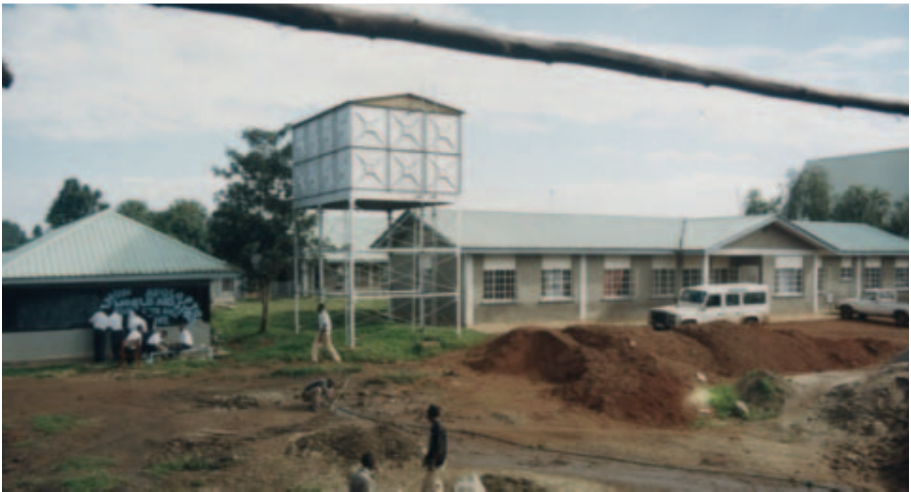
Renovations at the Canon Apolo Core Primary Teachers College in Uganda which were completed in 2003
